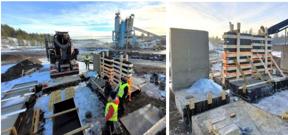
Figure 5.10. Overview of the large-scale testing site, Luleå, Sweden, October 2021 (photo credit: Trung Hieu Nguyen).
